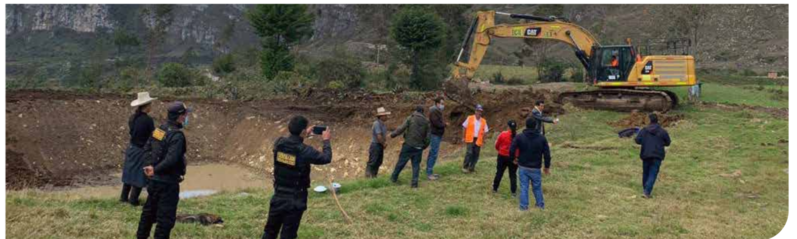
We partnered with authorities on the construction of small water reservoirs for agricultural purposes
